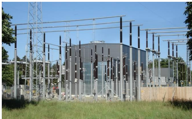
Figure 9. HVDC converter station at Lista
